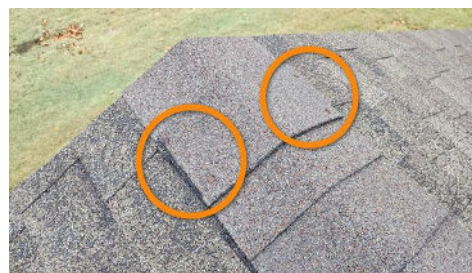
Shingle fasteners need sealed
