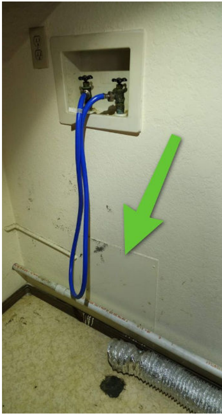
Below washer connections
