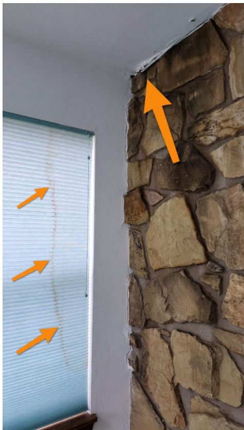
Evidence of moisture below gap
