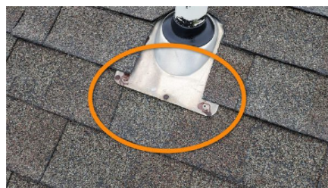
Flashing fasteners need sealed
