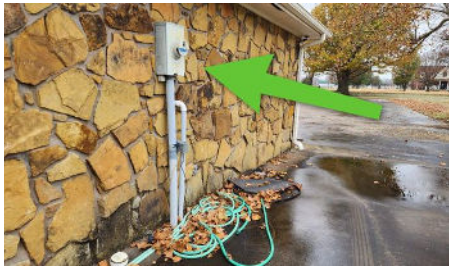
Service entrance/meter location
