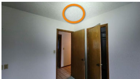
Missing in bedrooms
