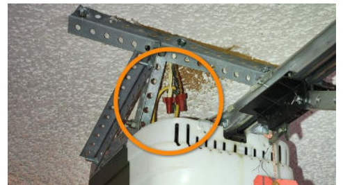
Garage door opener wiring
