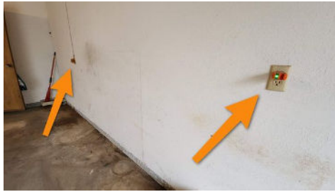
Needs gfc protection
