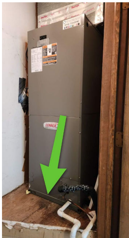
Filter located at base of air handler
