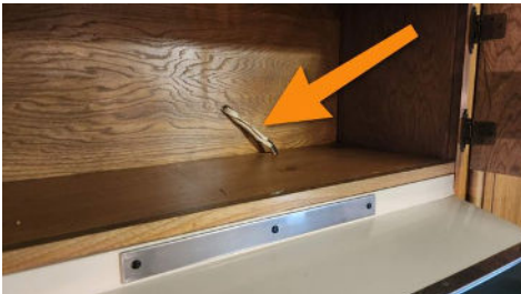
Above vent hood
