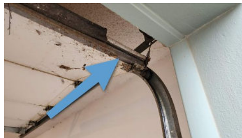
Damaged bottom seal
