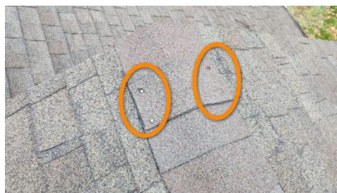
Shingle fasteners need sealed
