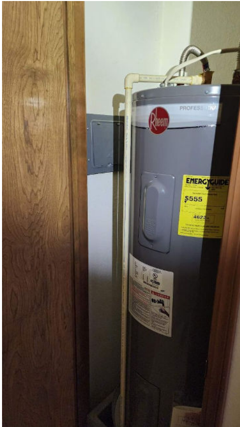
Inadequate work space clearance
