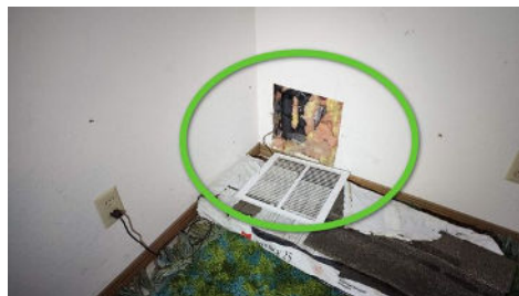
Repairs noted on inside wall
