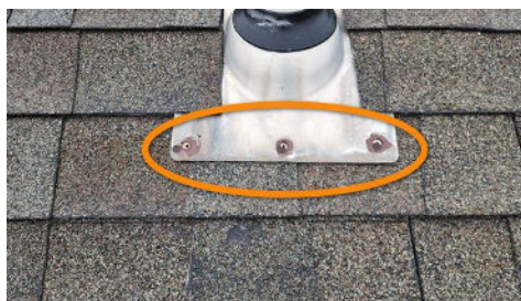
Flashing fasteners need sealed
