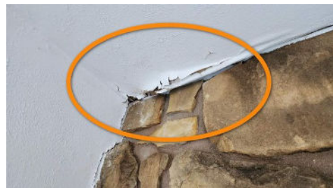
Moisture damage below this area
