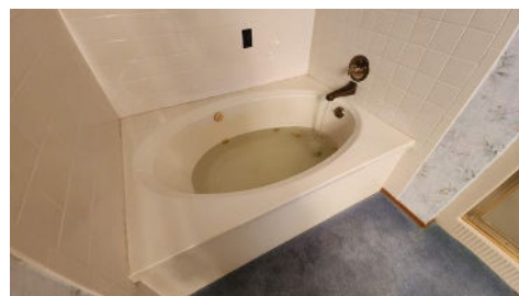
Hall bath/needs GFCI
