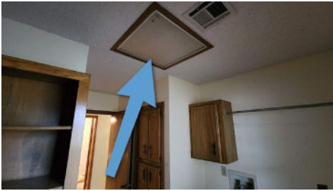
Laundry room light
