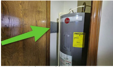
Sub panel location
