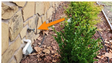
Front right exterior faucet
