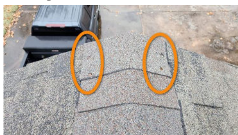
Shingle fasteners need sealed
