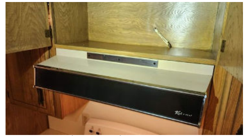
Not vented properly
