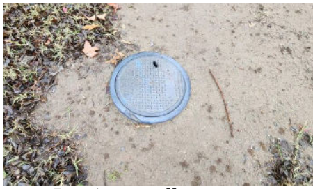
Exterior cut off at meter
