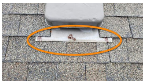
Flashing fasteners need sealed
