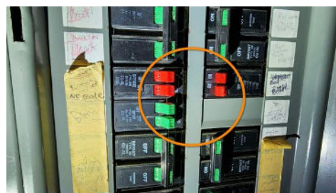
Missing handle ties
