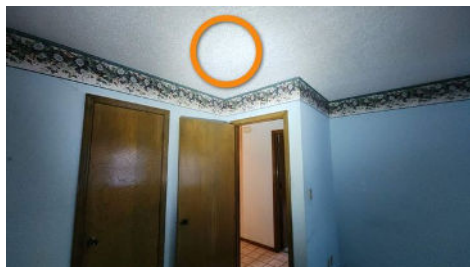
Missing in bedrooms
