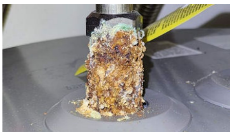
Heavy corrosion noted
