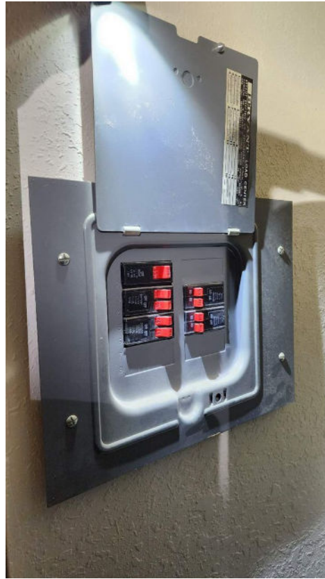
General sub panel photo
