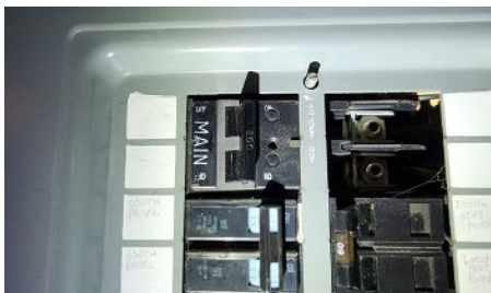
200 Amp main disconnect
