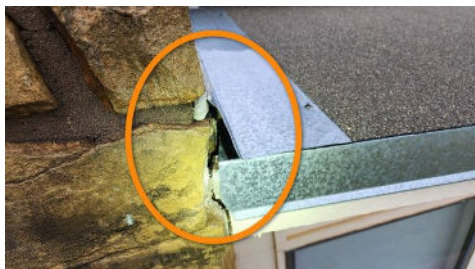
Gap in flashing
