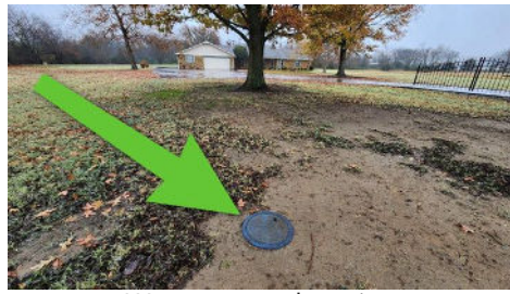
Water meter location
