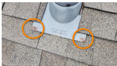
Flashing fasteners need sealed
